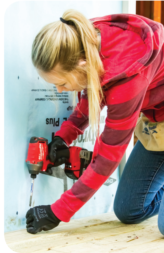
750 hours were contributed from our Truman Heritage Habitat for Humanity committee in building a new home. Many of our members on other committees also donated their time ( Total: 4,240 hours! ) to help the Schumacher family from Raytown, Mo., live in a safe, affordable home. Stephanie Sheldon uses a power drill to help build the Schumacher's front porch.
